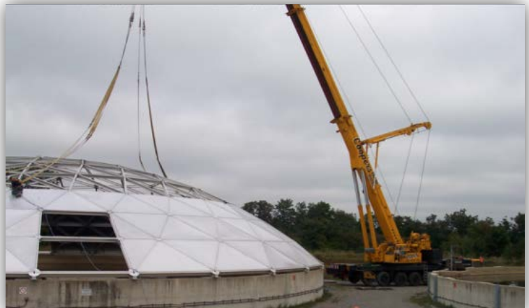
Greatario Engineered Storage Systems: An innovative solution at Halton included the construction of the dome in an adjacent field and then lifting it into place with a crane.
