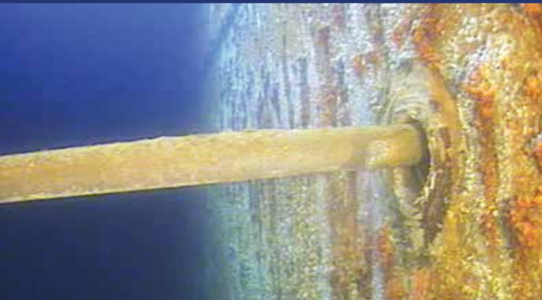
Corrosion discovered on tank panel
