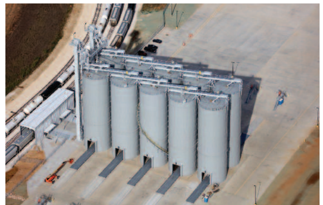
The chimed-panel, field-bolted steel silos shown here were constructed using the jack installation method, significantly reducing installation time.
