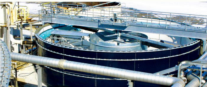
↑ Municipal Waste Water Clarifier/ Sludge/ Storage/Mixing
